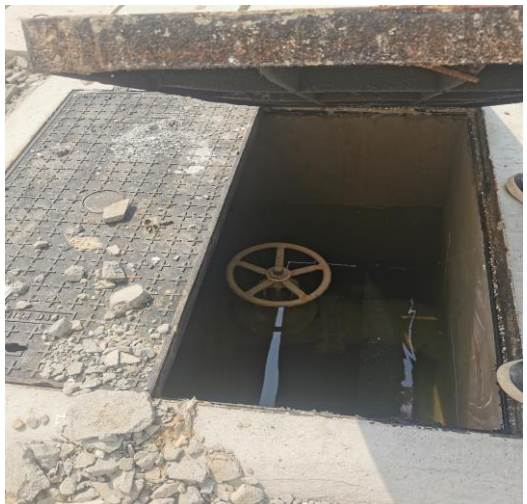
厂区污水总排口截断阀
